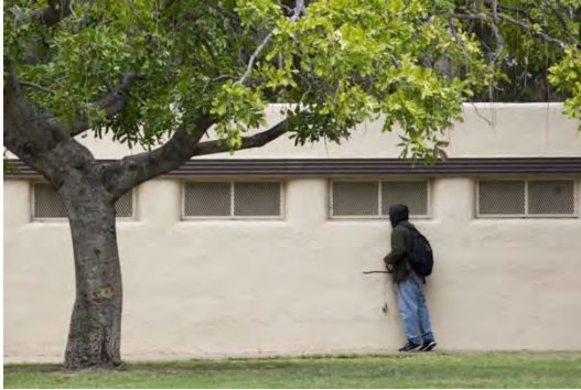
The public restrooms next to the San Diego Air and Space Museum in the Palisades area of Balboa Park were photographed on Wednesday in San Diego, California. A new report finds that all of Balboa Park's public bathrooms are in severe disrepair. (John Gibbins/The San Diego Union-Tribune)
