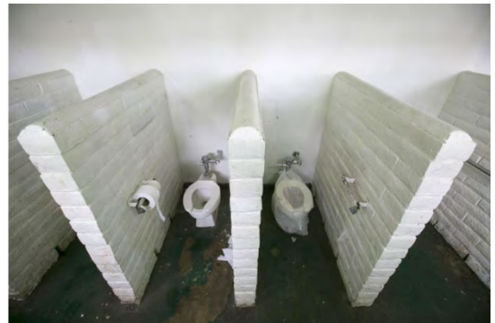
The inside of the public bathroom in the Palisades area of the park, next to the Air and Space Museum, as seen on May 8. (John Gibbins/The San Diego Union-Tribune)
