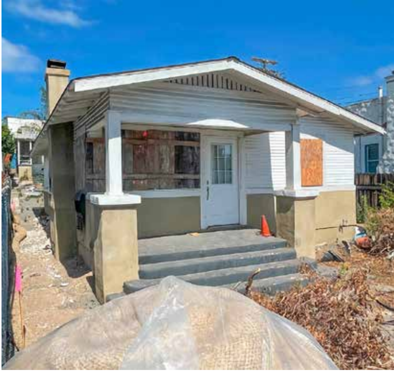
1925 Craftsman Bungalow at 4222 Georgia Street being torn down will be replaced by the Georgia Modern which features 5 stories, 31 units, and 2 parking spaces
